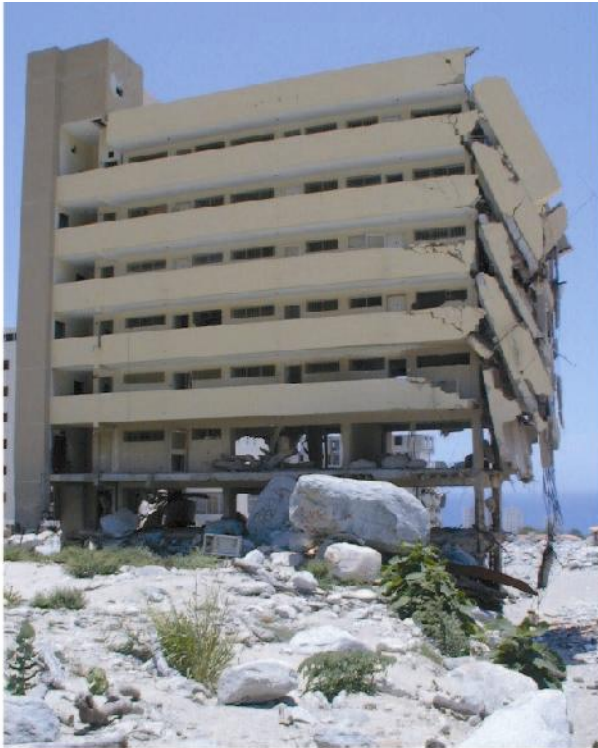
Figure 6. Apartment building damaged by debris flows, Caraballeda. Note collapsed apartments and boulders on floor of second story.
