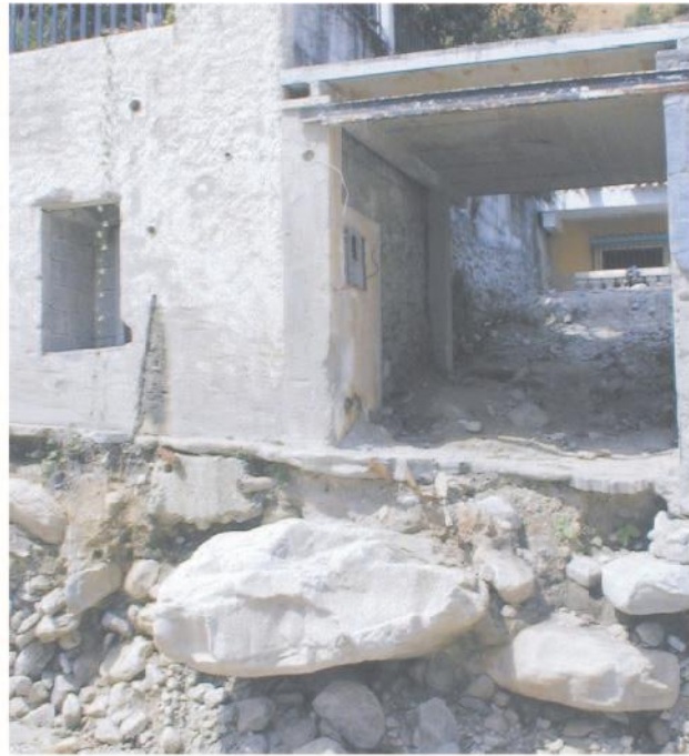
Figure 7. House and garage on Caraballeda fan with exposed foundation showing old debris flow deposit.
