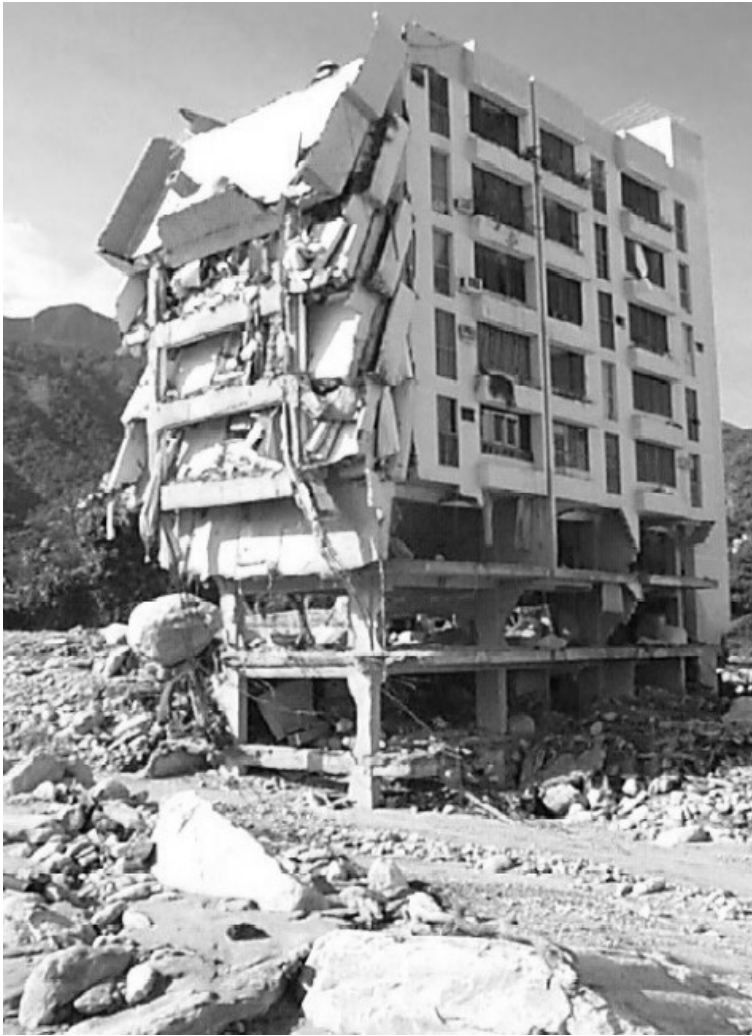
Figure 11. Flash-flood and debris flow damage to apartment building, Caraballeda, Venezuela. Note large boulder at level of second floor.
