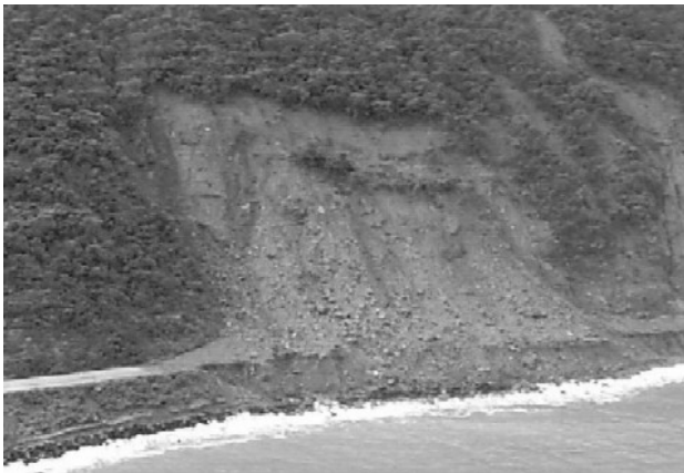
Figure 8. Landslide damage to two-lane coastal highway, Vargas state, Venezuela.
